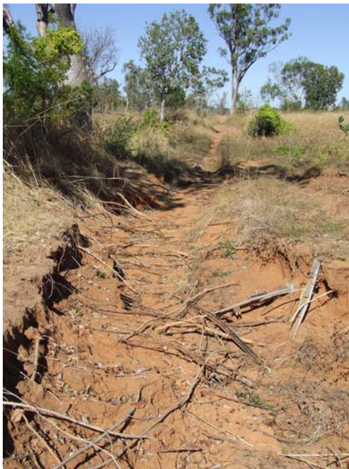
Figure 1: This fence line fire break has been eroded to the point that it has become a gully.
