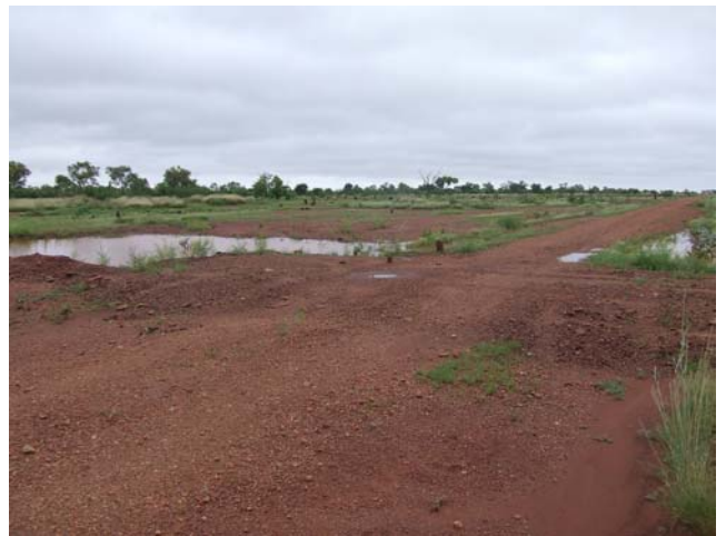
Figure 2: A roadway check bank, note the ponding of water in the sill on the left
